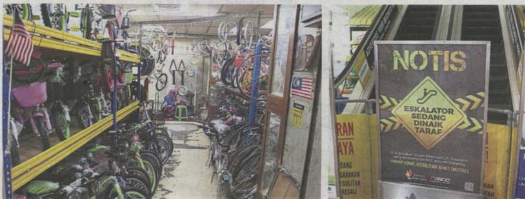
Escalators which have been out of order for some time will be replaced next year.
